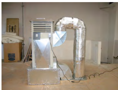
SolCool Unit on Mezzanine
